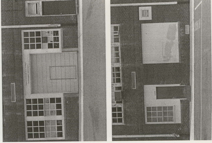
Figure 9. Two views of modified windows on the Fourth Street facade, lower level. (Preservation Piedmont)
